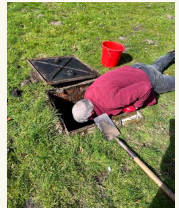
drainage system was given the once over. We found a broken manhole cover which was passed to the Council to repair.
